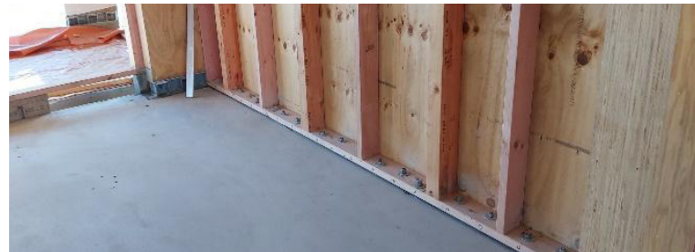
Fig. 32 - Photo showing plywood shear wall in which the chords are the LVL portal columns
