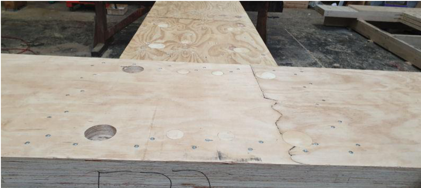
Fig. 17 - Bolt holes plugged with timber and sanded to an architectural finish in the TimberLab factory
